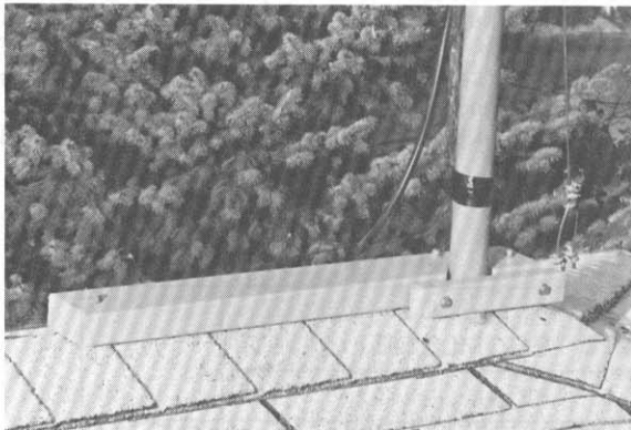
Fig. 10 — A V-cut 2 x 4 and screw-adjustable block make a roof-mounted mast clamp to prevent rotation. The roof was sealed before clamp installation. A heavy ground wire is attached to the mast for lightning protection. Dressed along the mast are coaxial and rotator control cable, which has been wrapped with grounded copper mesh to prevent RF pickup from feeding the shack.
